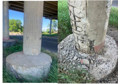
Fig. 11: Destruction of the protective layer of concrete, exposure of reinforcement, destruction of the concrete slab
