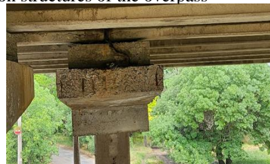
Fig. 7: Unsatisfactory condition of the concrete of the ends of the supporting beams
