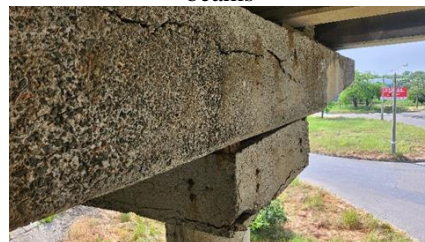
Fig. 9. Destruction of the protective layer of concrete of the support beam
