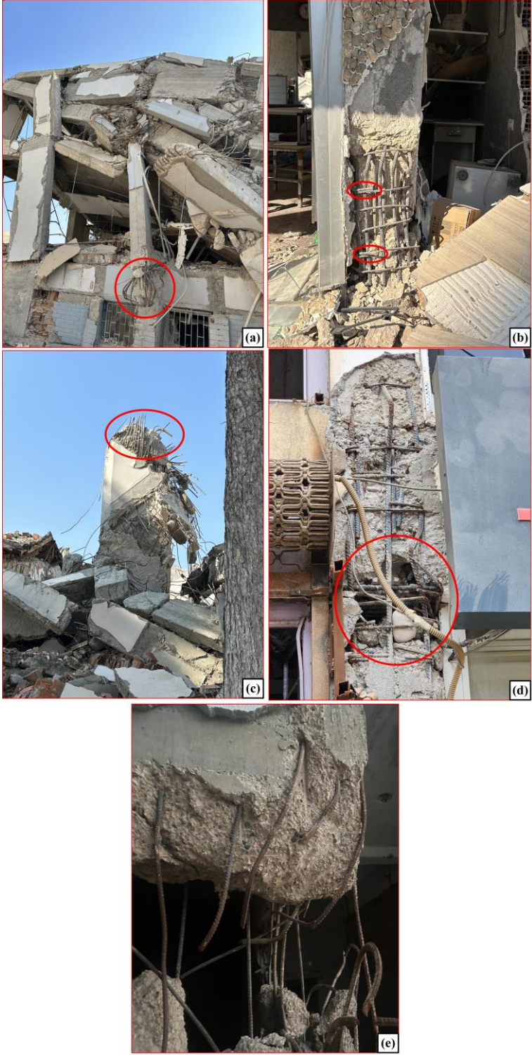
Figure 3: Damages Related to Reinforcement Detailing and Material Grades
