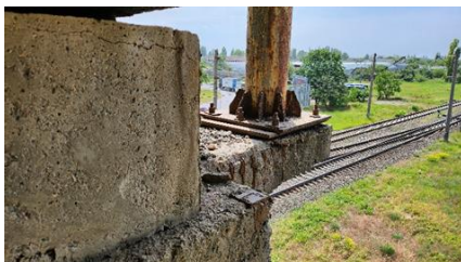
Fig. 8. Unsatisfactory condition of consoles under street lighting lamps
