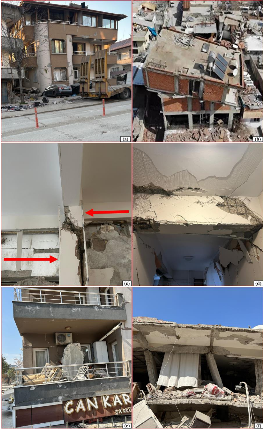
Figure 4: Damages Related to Structural System Deficiencies
