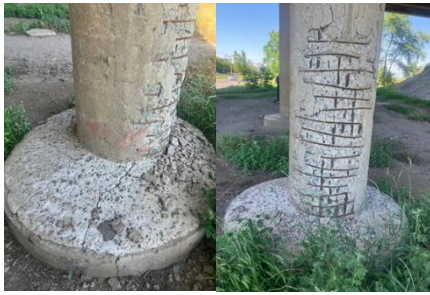
Fig. 10: Destruction of the protective layer of concrete, exposure of reinforcement, destruction of the concrete slab
