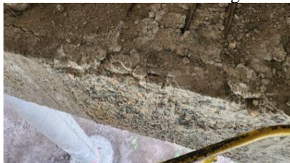
Fig. 6: Destruction of the concrete of the monolithic section of the support beam
