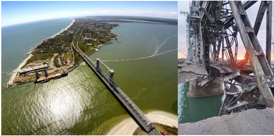
Fig. 2: The destruction of the bridge structures in the Zatoka village of Odesa region because of numerous rocket attacks
